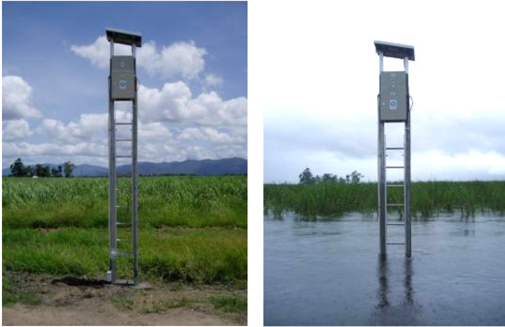
Figure 8 S2 sampling system installed at location 07 on the Murray River floodplain.
