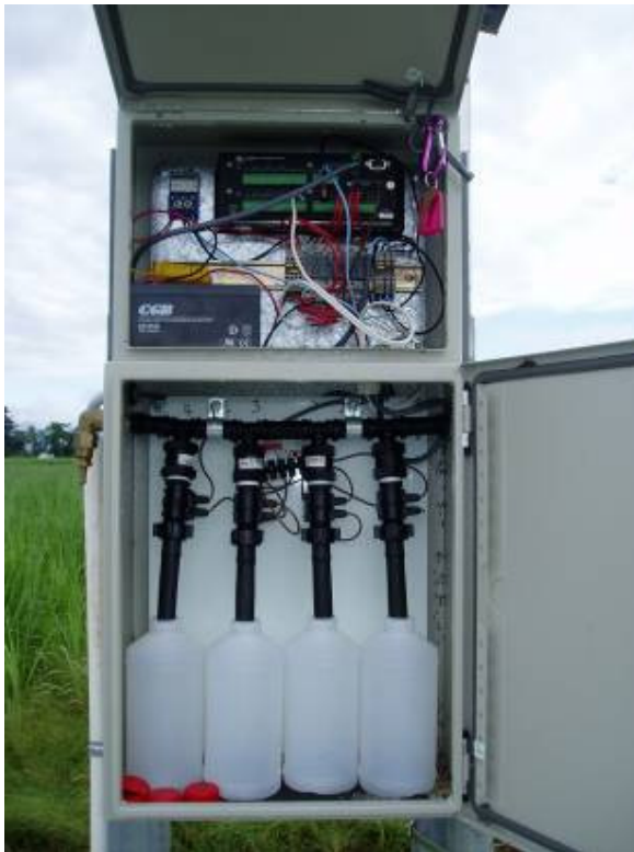
Figure 10 Components of the S2 sampling system.
