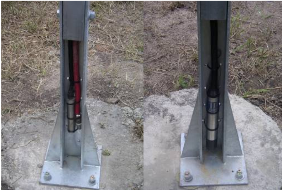
Figure 6 Turbidity probe and auto-sampler intake (left) and depth sensor (right) mounting positions.
