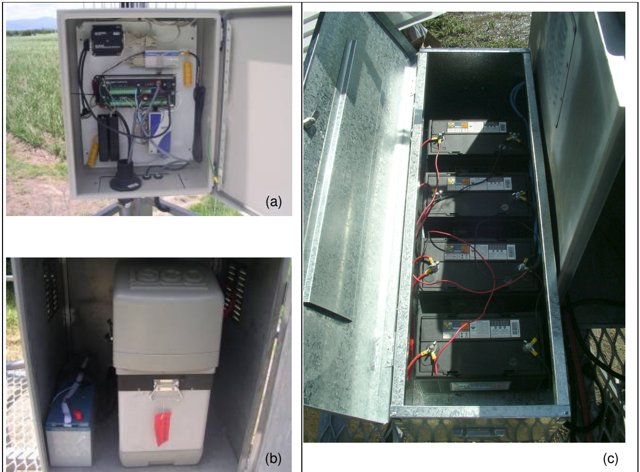
Figure 5 Logger enclosure (a), auto sampler enclosure (b) and battery enclosure (c).
