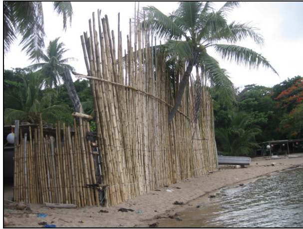
Figure 5: The bamboo wind break constructed out the front of an Erub Island Aunty's property. Photo by Karen McNamara.
