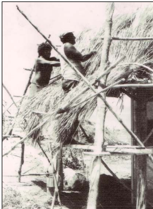
Figure 6: Erub Islanders building a traditional house using grass materials for the roof. Photo extracted from Erub Island Council Library records.
