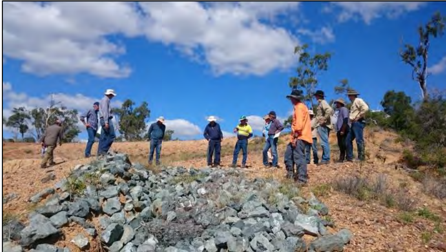
Failed rock chute, undermined by collapsing dispersive soils.
