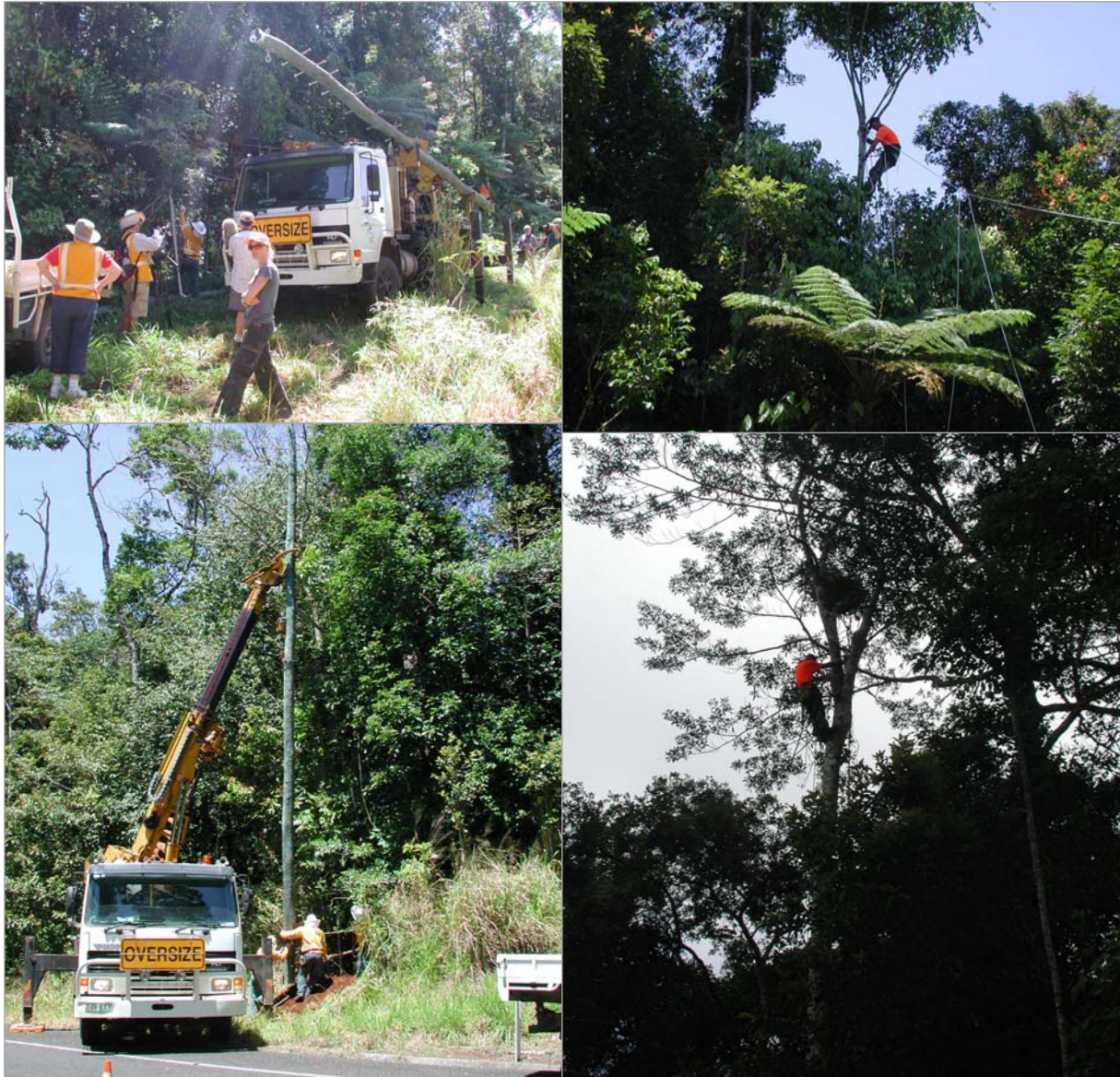
Figure 2.4 Canopy bridges were installed between an electricity pole on one side of the road and a large, solid, healthy tree on the other side. Photos courtesy of Birgit Kuehn.
