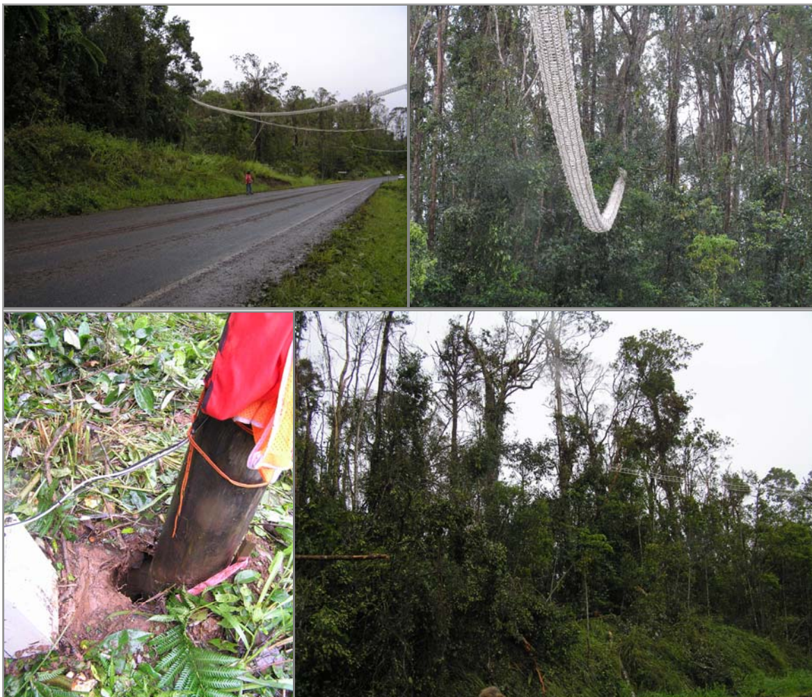
Figure 2.15 Photographs taken three days after category 4 Tropical Cyclone Larry passed almost directly over the Palmerston Highway and its canopy bridges. The bridges are still in place although with slight sagging of the rope tunnel, a pole loosened in ground, and damage next to one of the ladders. Photos courtesy of Steve Goosem.
