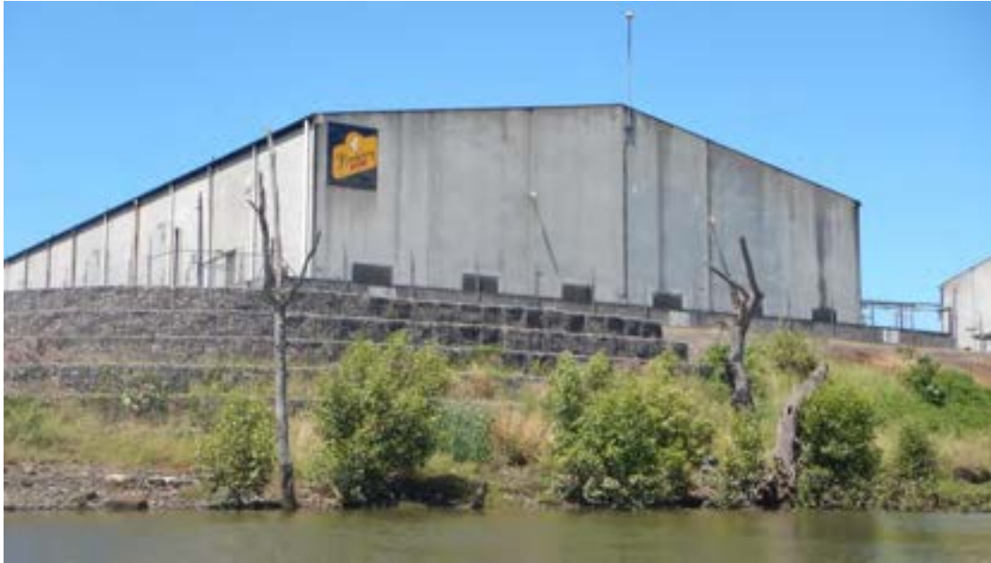
Figure 110: Bank hardening has been undertaken without regard for tidal wetlands or riparian margins in many areas bordering the Burnett estuary.
