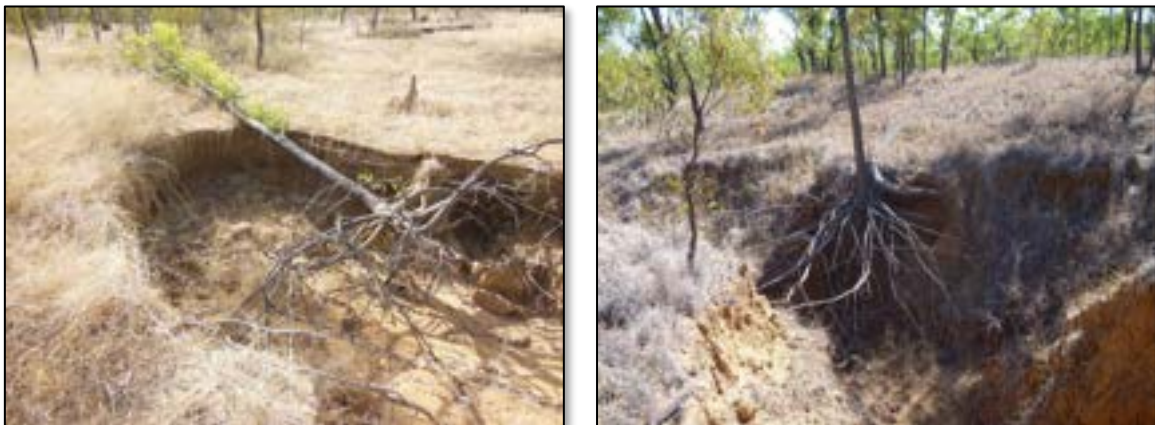
Figure 52: Examples of root exposure with very recent erosion activity and head retreat evident.
