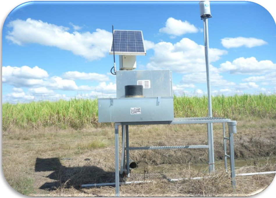
Figure 7. Instrumentation for the collection, measurement and sampling of run-off from the end of the furrow irrigation block in the sugarcane trial block on a heavy clay soil, Clare, Burdekin.
