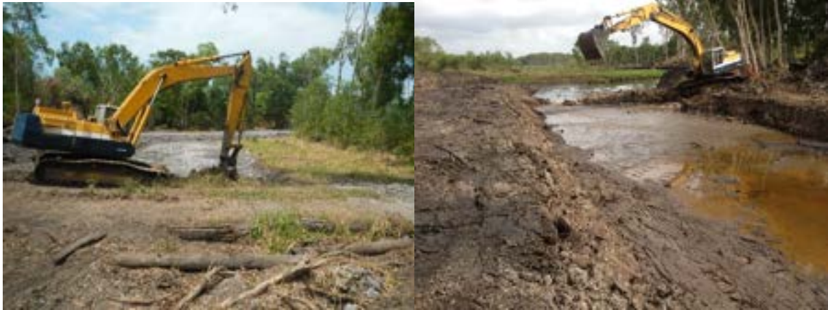
Figure 3: Excavator breaching the earth wall in August 2013 (Photo credits M. Nicholas)
