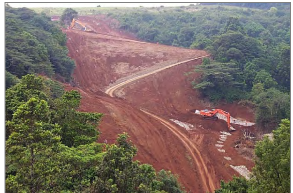
Changes in runoff, stream flow and sedimentation can be of a large scale: the sediment trap constructed as part of this upgrade failed following heavy rainfall during the tropical monsoon period, releasing sediment into nearby streams and waterways.
